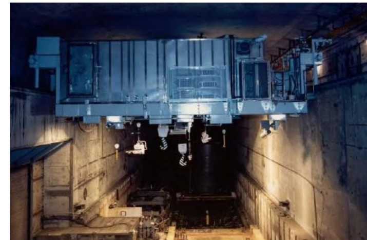
H-Canyon Overhead Crane
