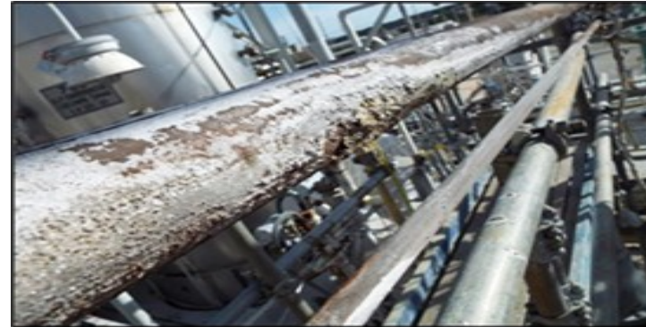
Corroded/Failing Caustic Header
