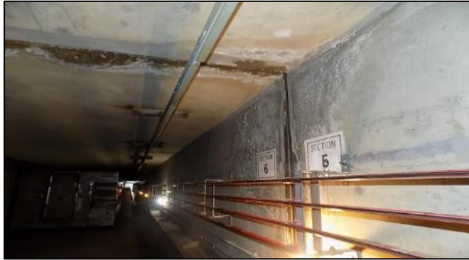
221-H Hot Crane Runway/ Power Rails with Water Intrusion Shown
